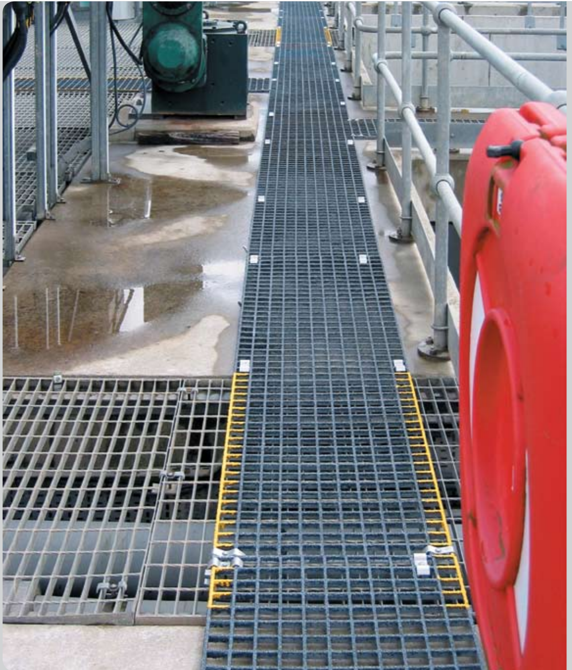
Water treatment plant
